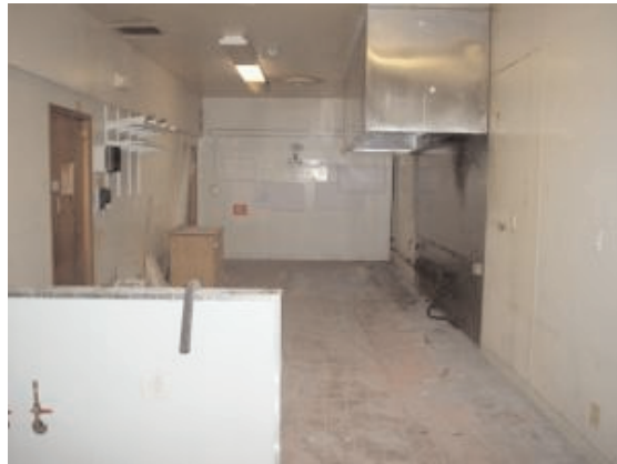
Kitchen has plumbing, venting & electric in place for a commercial kitchen. Also has an ansef fire suppression system.
